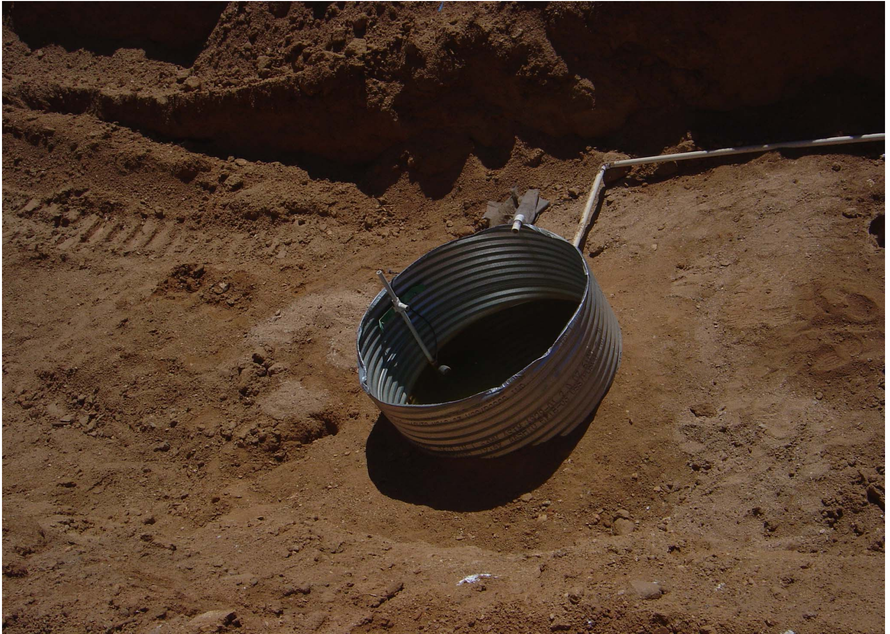
PHOTO 4–Five Foot Diameter Stand Pipe
