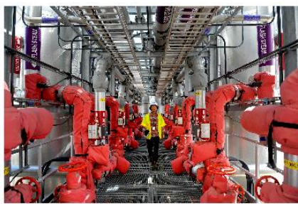
Ryu Suzuki, an engineer at the new Bailey Bioenergy Facility, walks past the state-of-the-art machinery that creates thermal hydrolysis. (Katherine Frey/The Washington Post)
