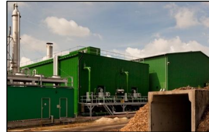
Rijsenhout (NL) Recovering CH 4 and CO 2 for greenhouses
