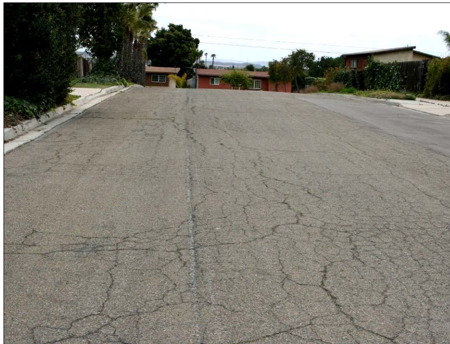
Figure 3.6 PCI = 40 (Poor Condition)
