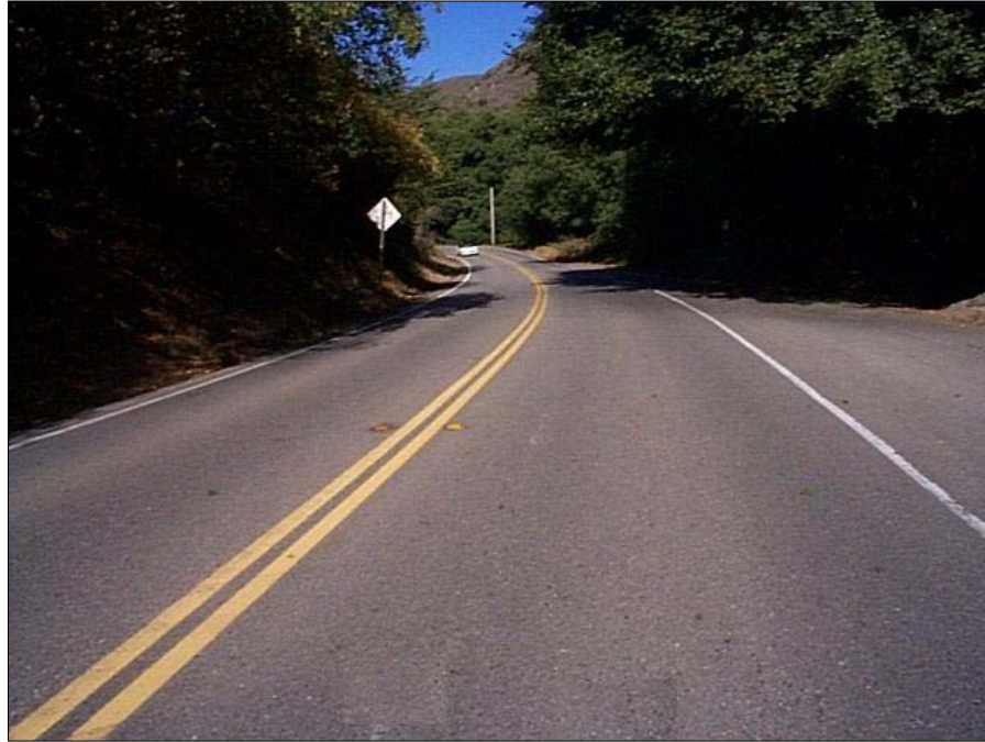
Figure 3.3 PCI = 98 (Excellent Condition)
