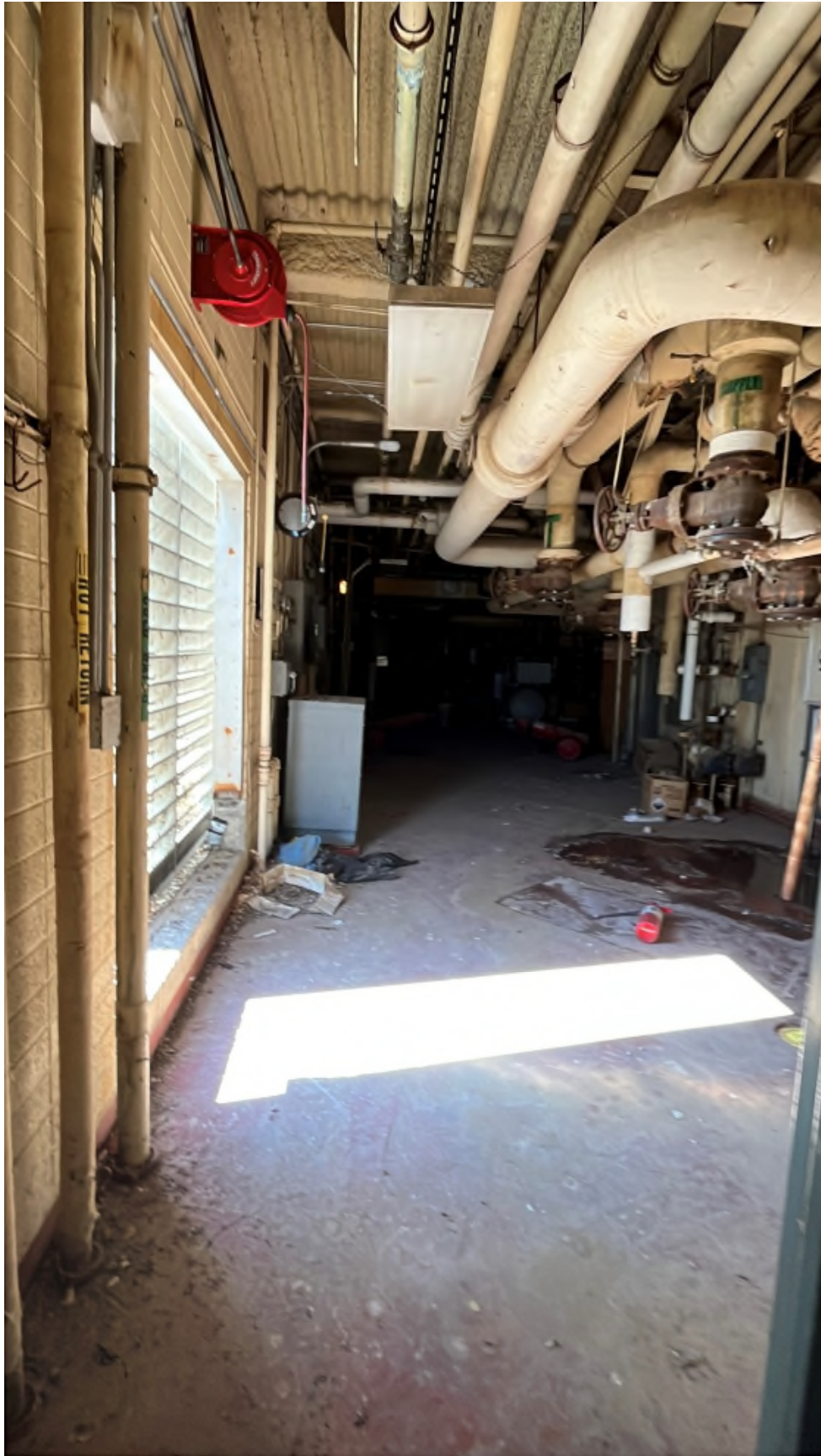
Mechanical Room Picture #1
