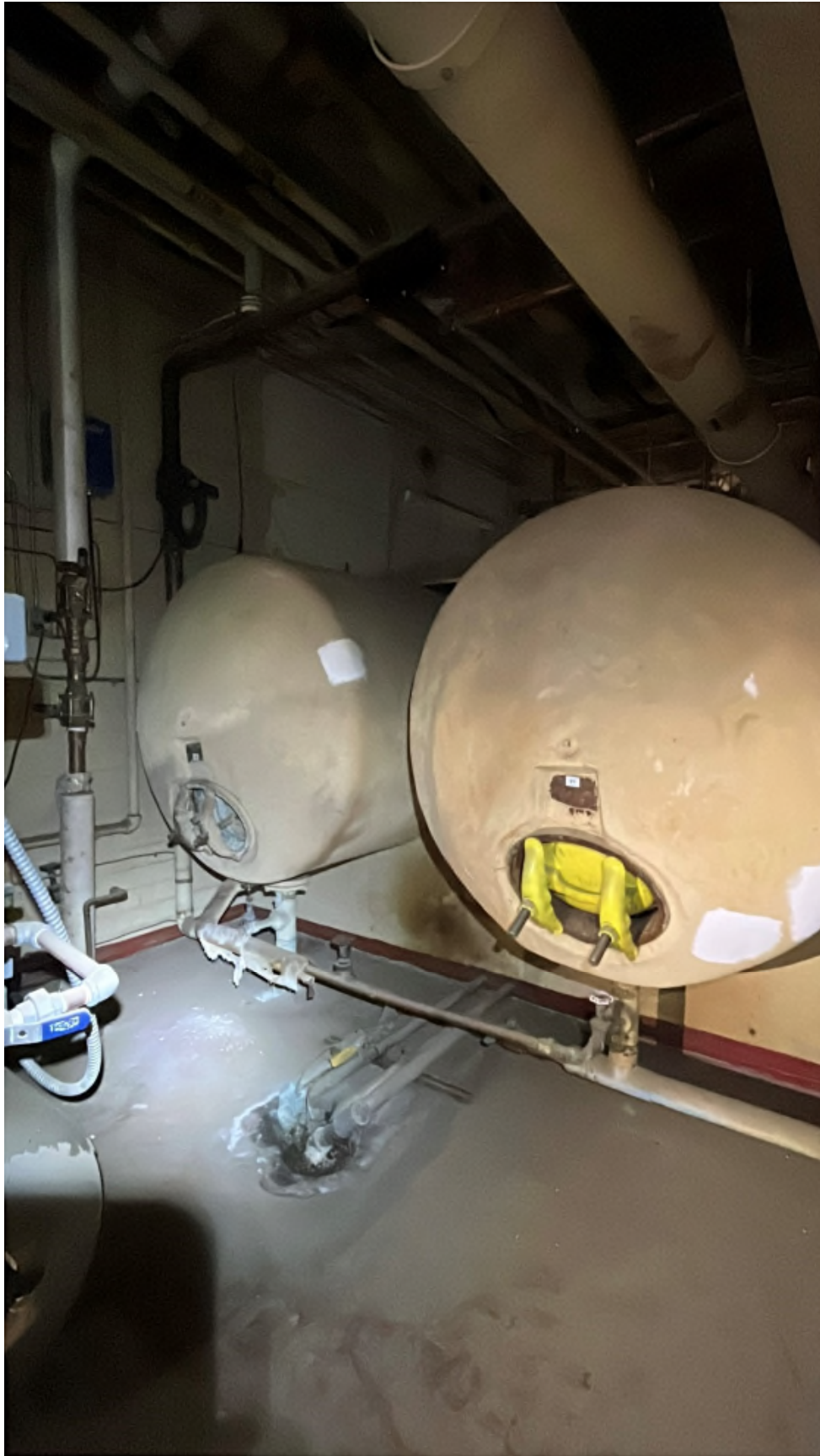
Boilers in Mechanical Room
