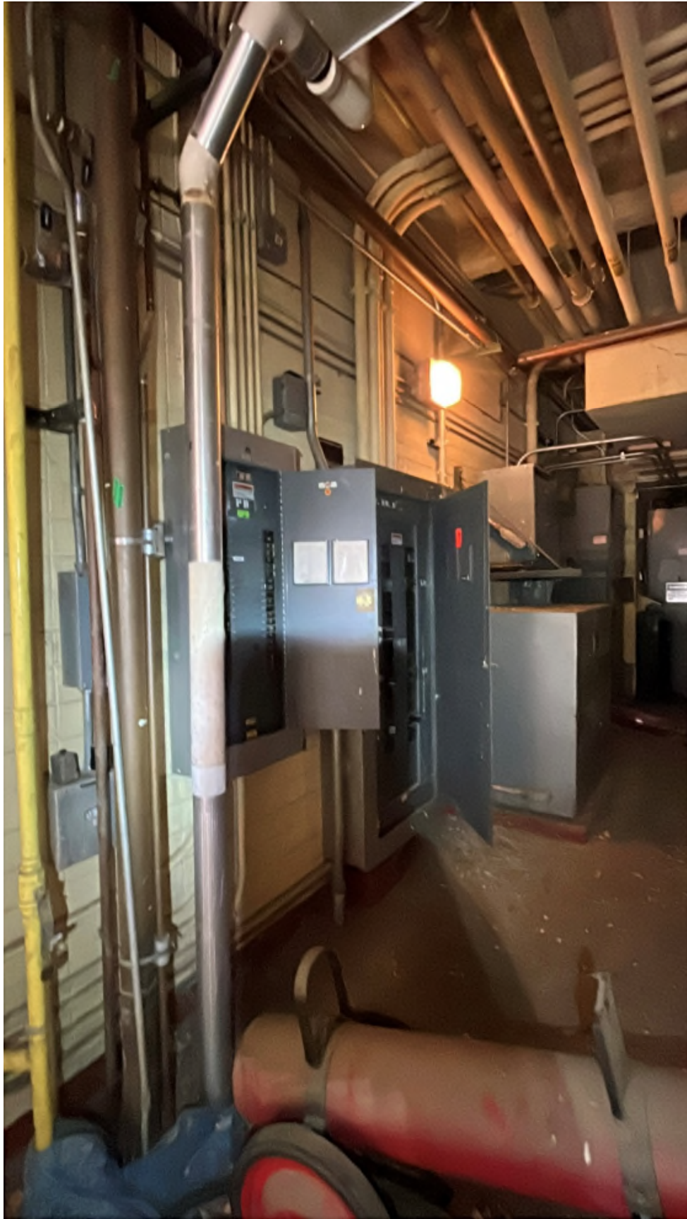
Mechanical Room Picture #5
