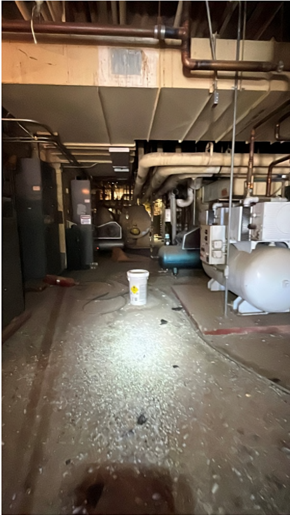
Mechanical Room Picture #7
