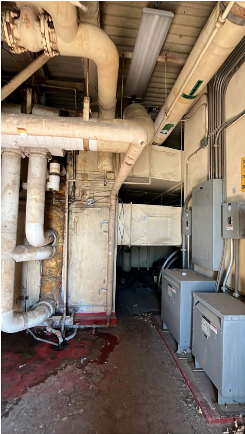
Mechanical Room Picture #2
