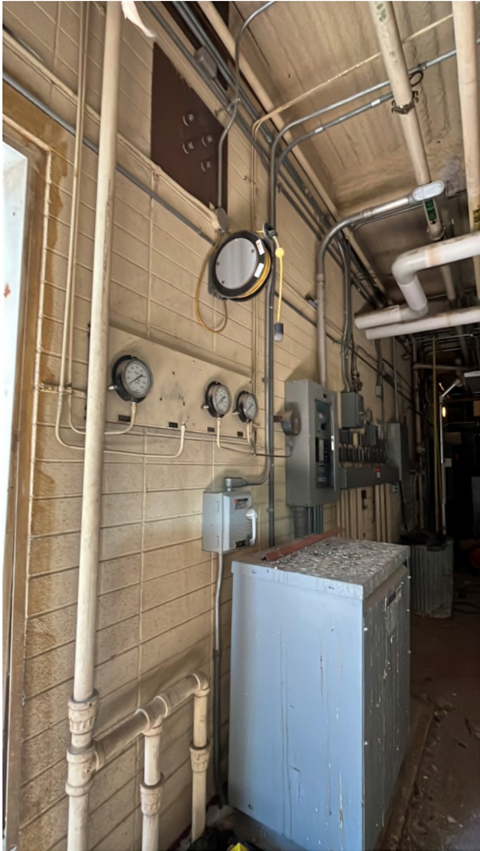
Mechanical Room Picture #4
