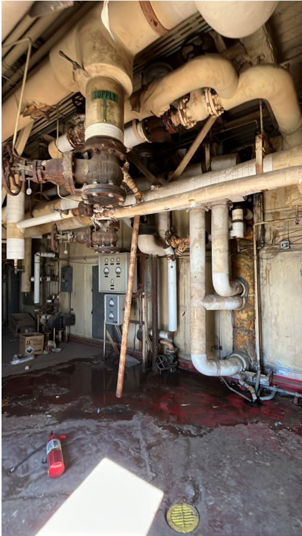
Mechanical Room Picture #3
