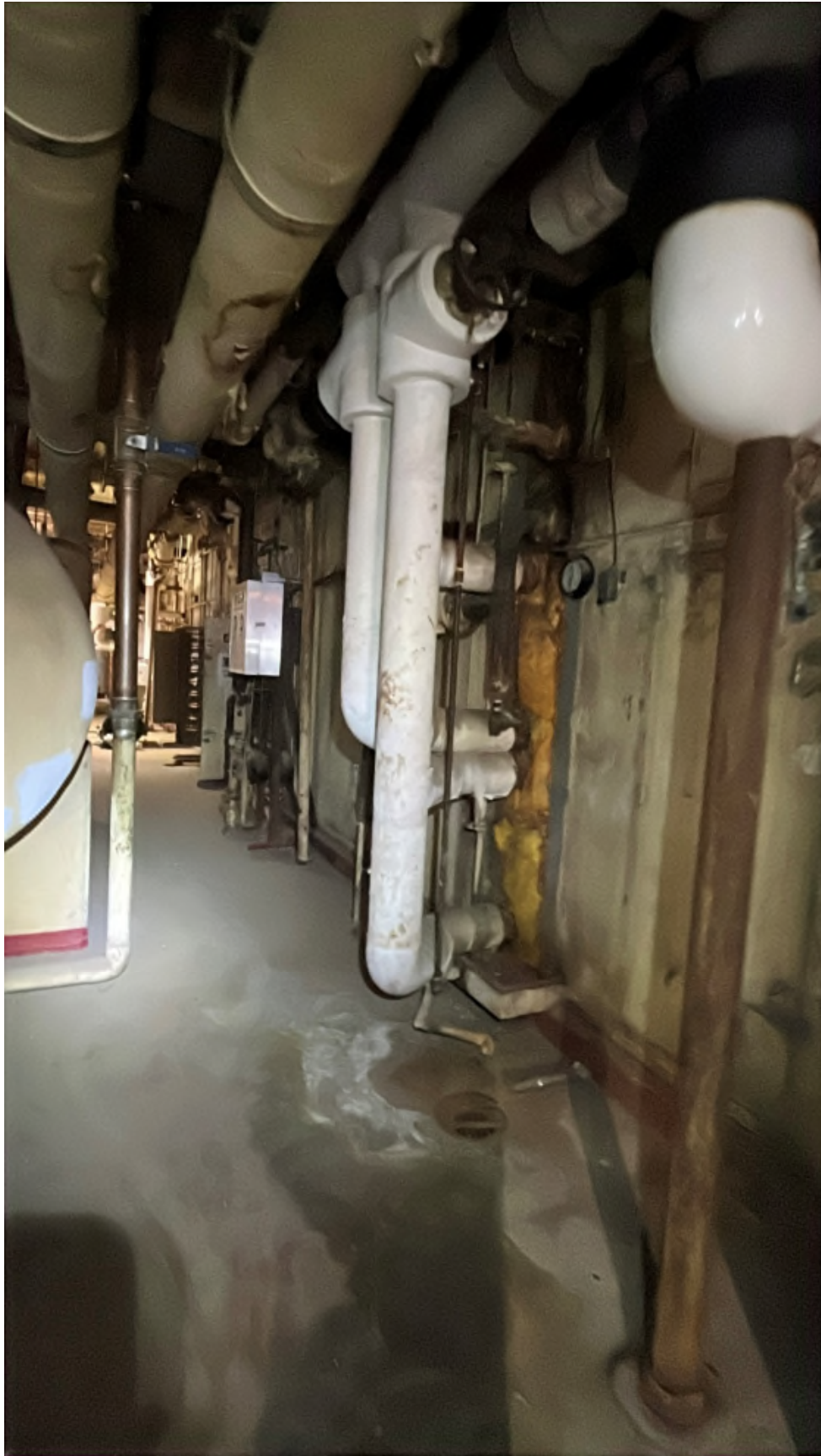
Mechanical Room Picture #9
