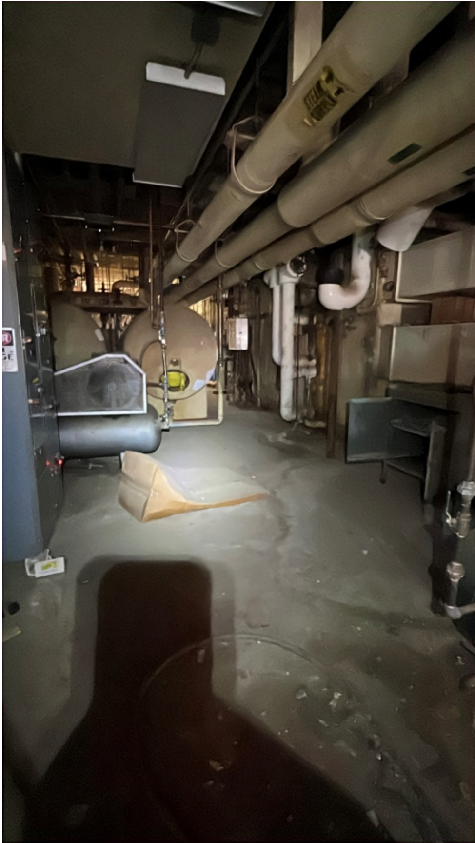
Mechanical Room Picture #8
