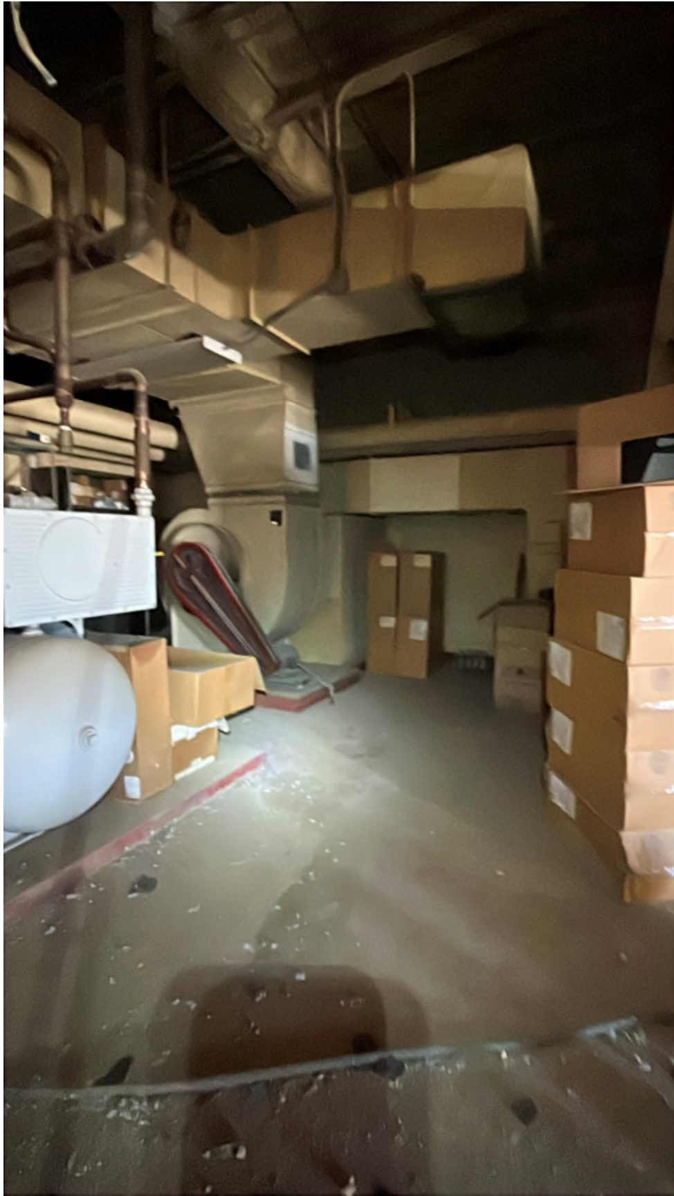
Mechanical Room Picture #6
