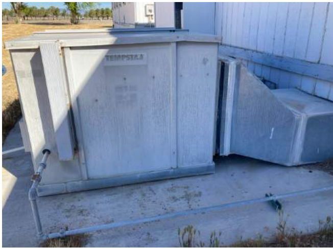
View of HVAC
