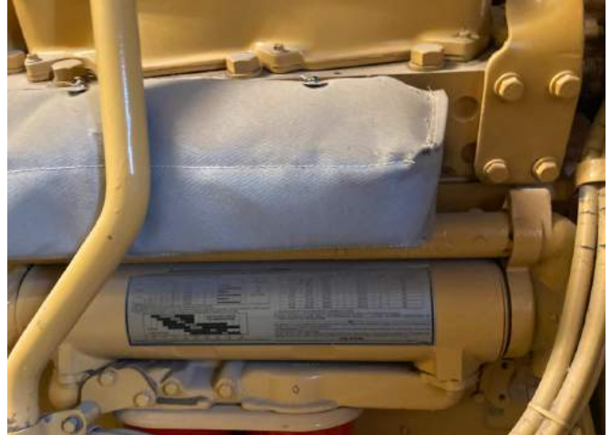
View of Generator Label
