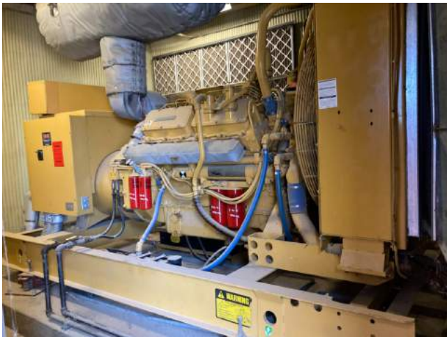
View of Generator
