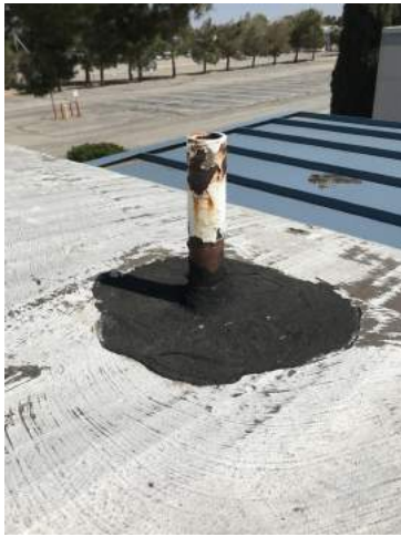
View of Penetration Mastic
