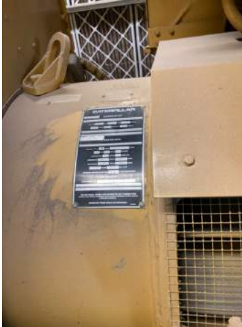
View of Generator Label
