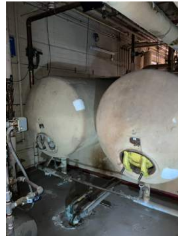
View of Large Boilers in Mechanical Room
