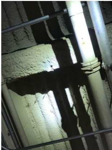
View of Fireproofing
