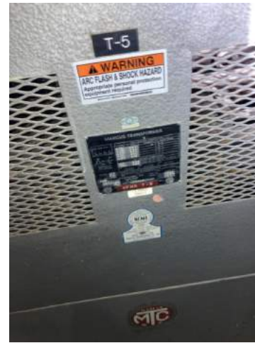
View of Transformers
