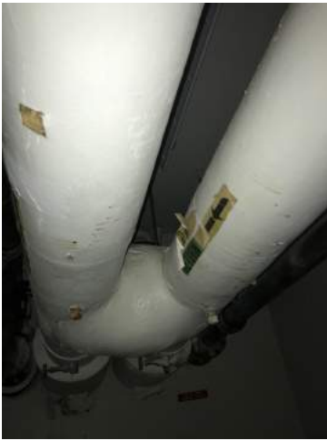
View of 4" Thermal System Insulation Pipe Run Wrapped in Foil
