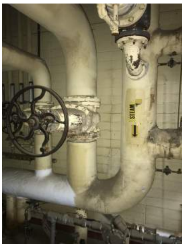
View of 4" Thermal System Insulation Pipe Elbows/Runs
