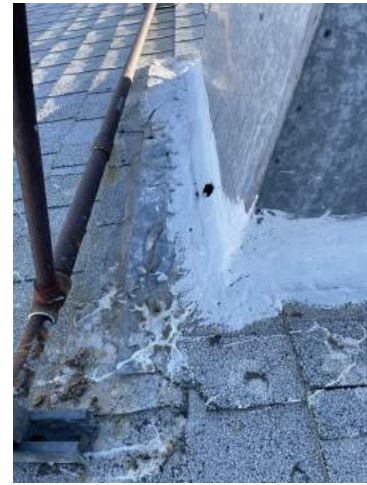
View of Penetration Mastic
