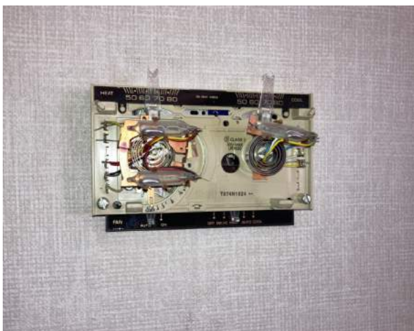
View of Mercury Switch
