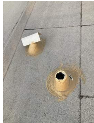
View of Brown Penetration Mastic
