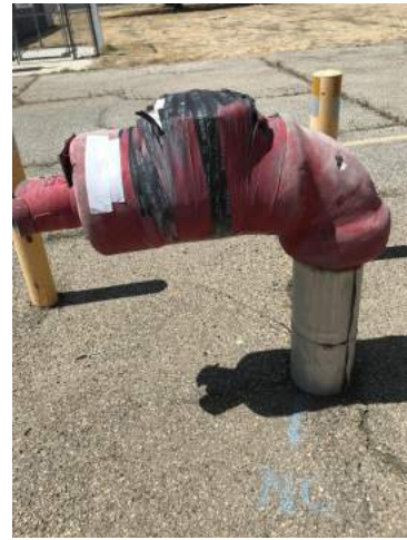
View of Red Laced Pipe Insulation
