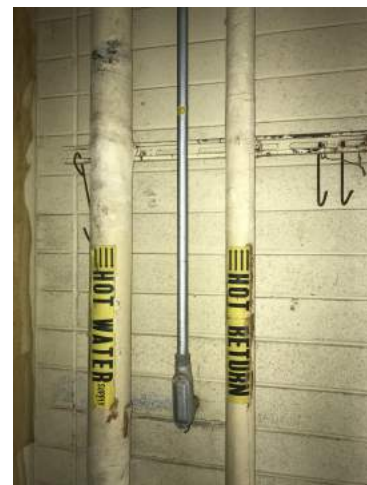
View of 2" Thermal System Insulation Pipe Elbows/Runs
