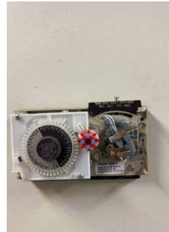
View of Mercury Switch
