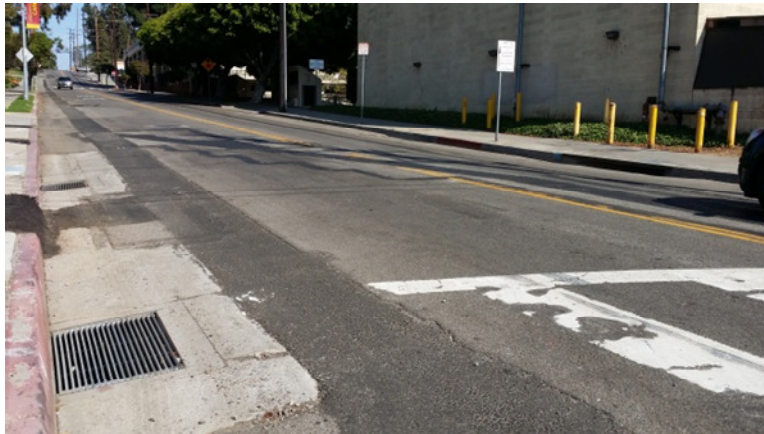
Photo 18: Storm Drain Inlet Along Zonal Avenue at Biggy Street Intersection
