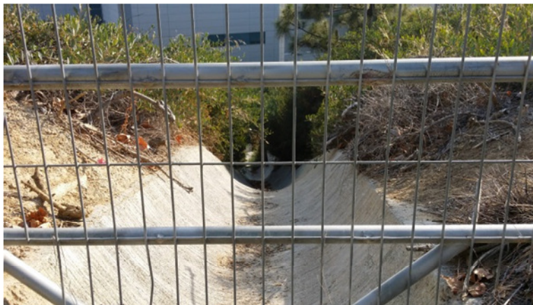
Photo 62: Looking at Concrete Conveyance Swale Running Perpendicular to Slope of “the Hill” in Northeastern Portion of Site
