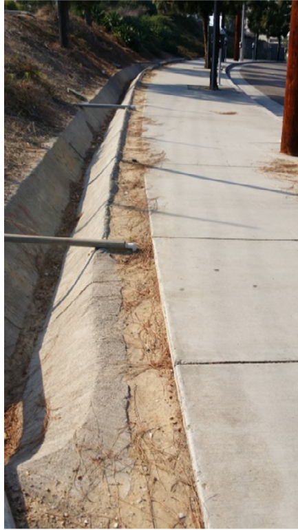
Photo 57: Looking at Concrete Conveyance Swale Along Cornwell that Flows Perpendicular to Slope of “the Hill” in Northeastern Portion of Site
