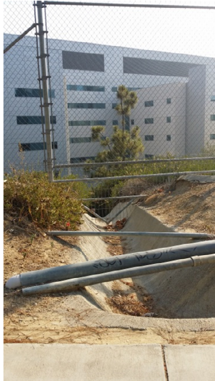
Photo 59: Looking at Concrete Conveyance Swale Running Perpendicular to Slope of “the Hill” in Northeastern Portion of Site
