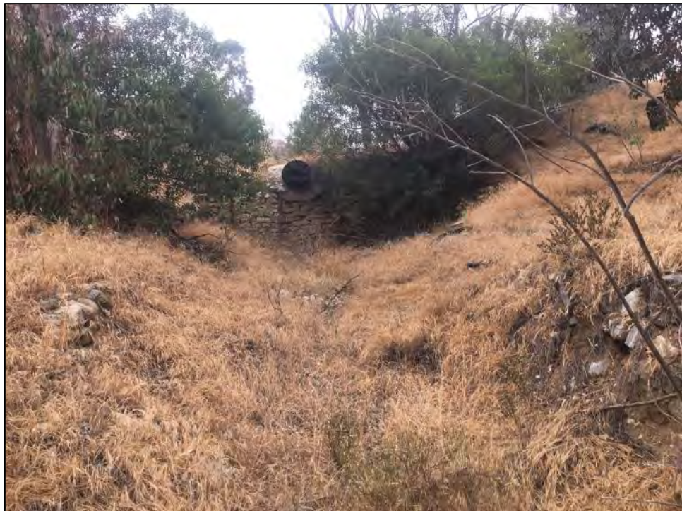
Figure 7. Area mapped as Pacoima Formation (Qp) showing grading disturbances and an installed artificial drainage.
