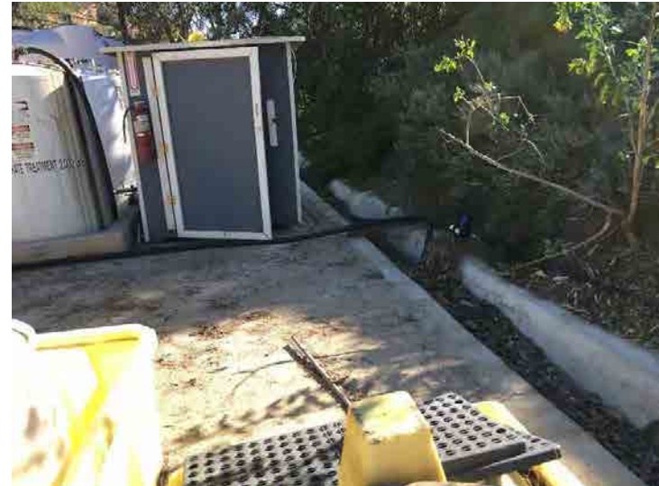
Photo 498: Leachate Treatment Facility: February 24, 2016
