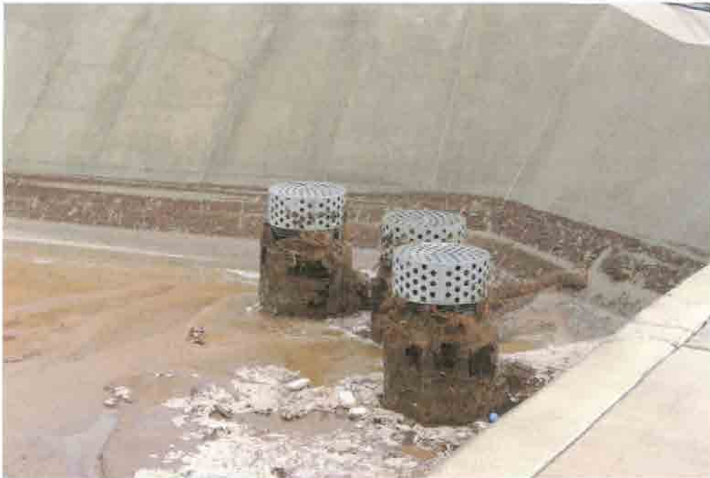
Figure 4: Risers in Terminal Basin
