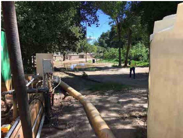
Photo 507: Gray Water Treatment & Handling Facility: March 9, 2016
