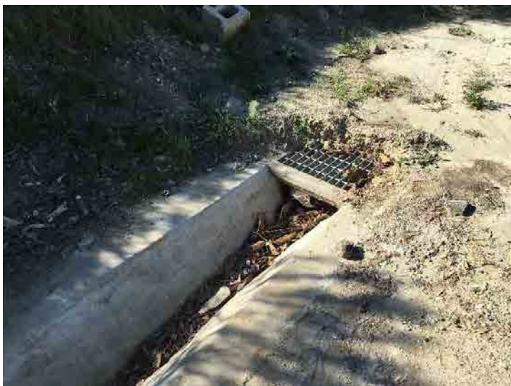
Photo 499: Leachate Treatment Facility: February 24, 2016
