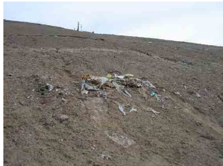
Photo 332: County South Slope Inert Waste Exposed: January 27, 2016
