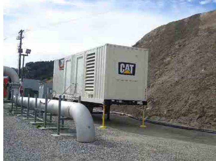
Photo 156: 35 Flare 9 & 10 Portable Generator: January 27, 2016
