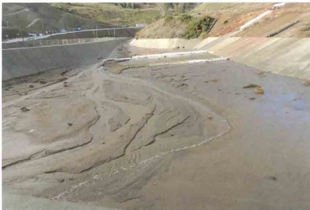
Photo 2: Sediments accumulation in terminal basin
