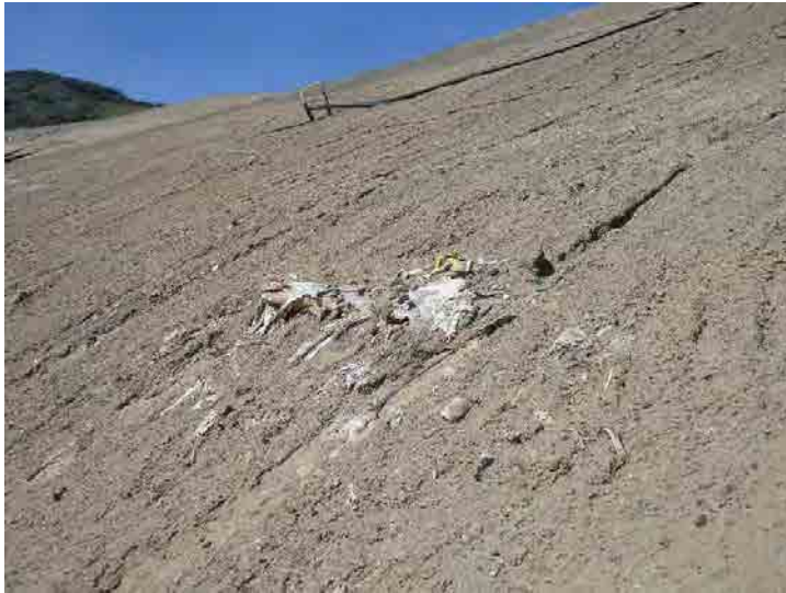
Photo 357: City Slope Erosion, Inert Waste Exposed: February 24, 2016
