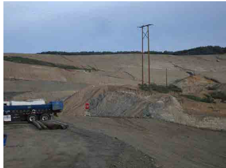
Photo 336: County South Slope Erosion Control: January 27, 2016
