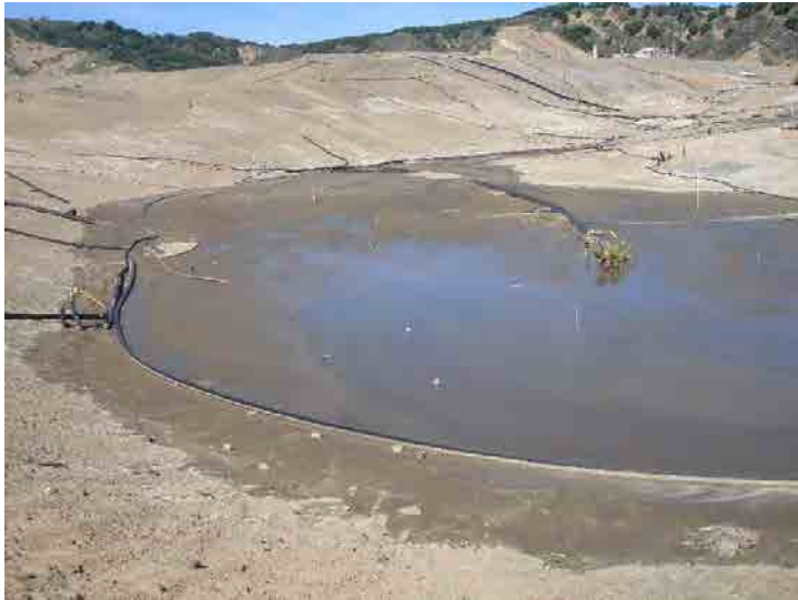
Photo 365: Ponding on City Top Deck: March 9, 2016
