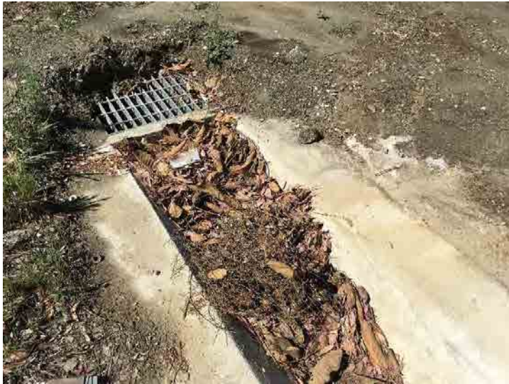
Photo 505: Leachate Treatment Facility: March 9, 2016
