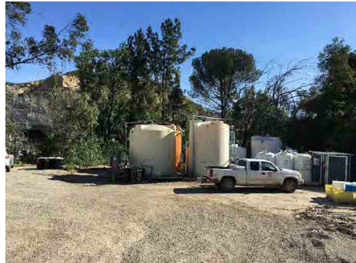
Photo 496: Leachate Treatment Facility: February 24, 2016
