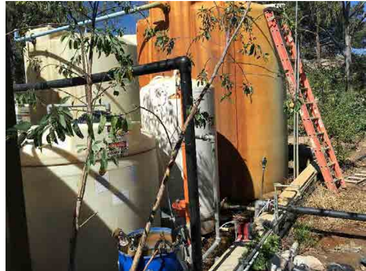
Photo 502: Leachate Treatment Facility: March 9, 2016
