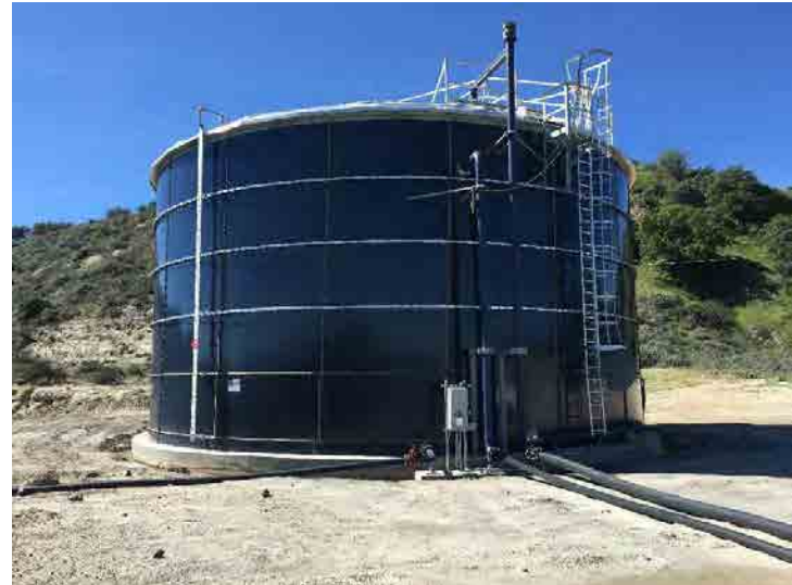
Photo 494: New Facility Water Tank: March 9, 2016
