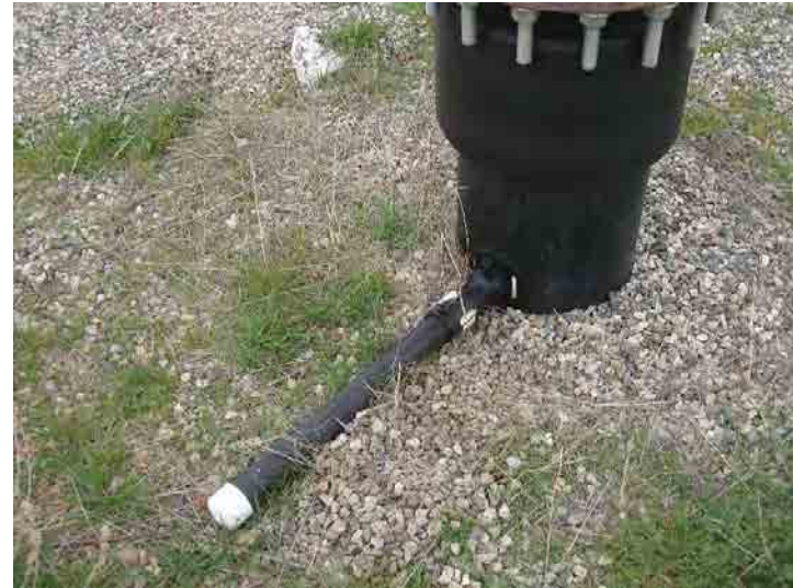
Photo 158: Flare 8 Vacuum Leak: January 27, 2016
