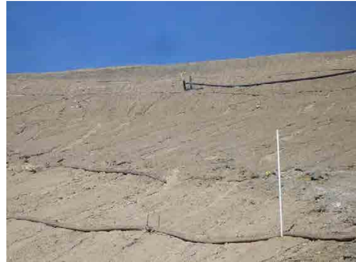
Photo 354: City Slope Erosion: February 24, 2016
