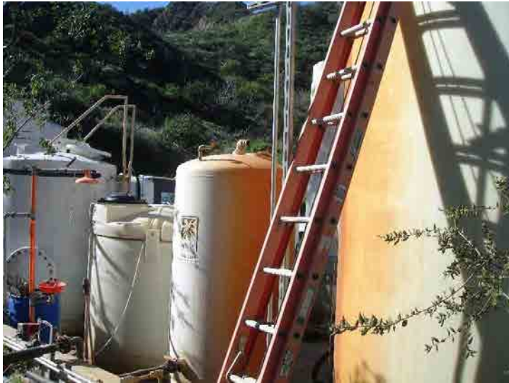
Photo 497: Leachate Treatment Facility: February 24, 2016
