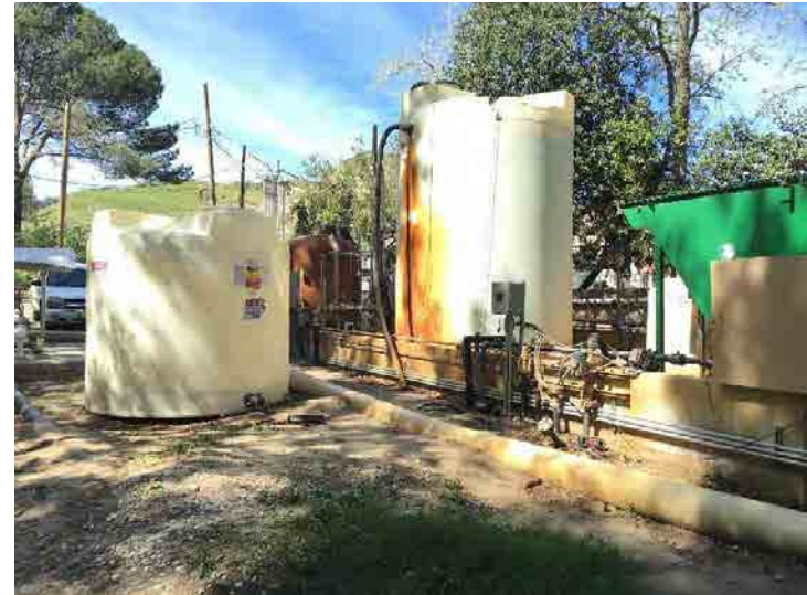
Photo 506: Gray Water Treatment & Handling Facility: March 9, 2016
