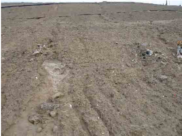
Photo 331: County South Slope Inert Waste Exposed: January 27, 2016
