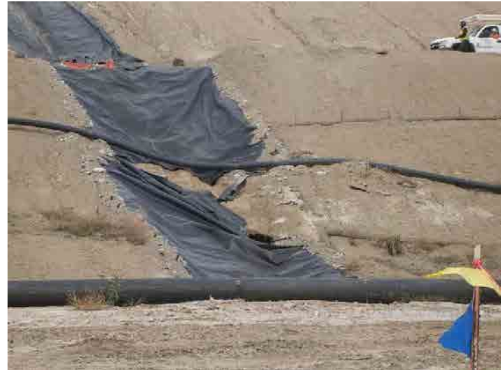
Photo 330: County South Slope Drainage Failure: January 27, 2016
