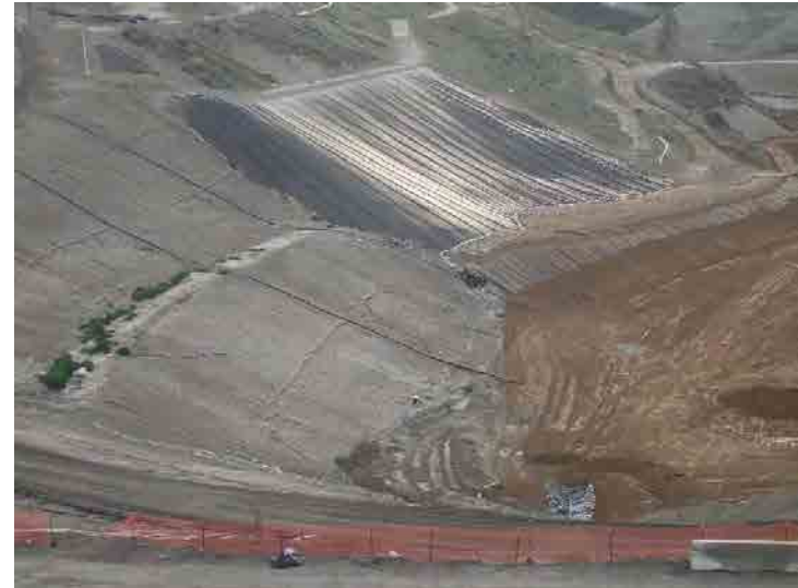
Photo 346: City Slope Erosion Control: January 27, 2016
