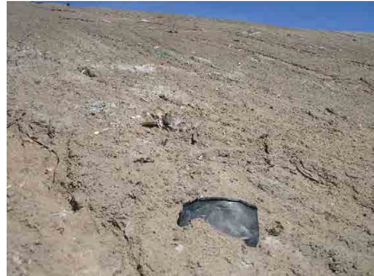
Photo 358: City Slope Erosion, Inert Waste Exposed: February 24, 2016
