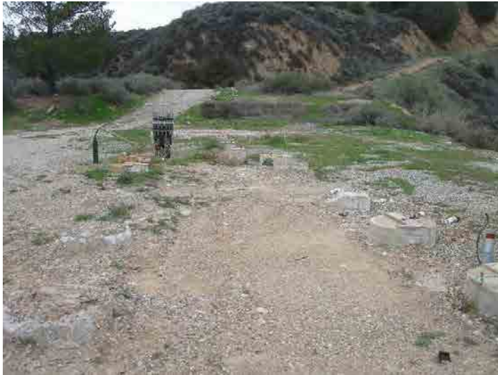
Photo 157: Flare 8 Vacuum Leak: January 27, 2016
