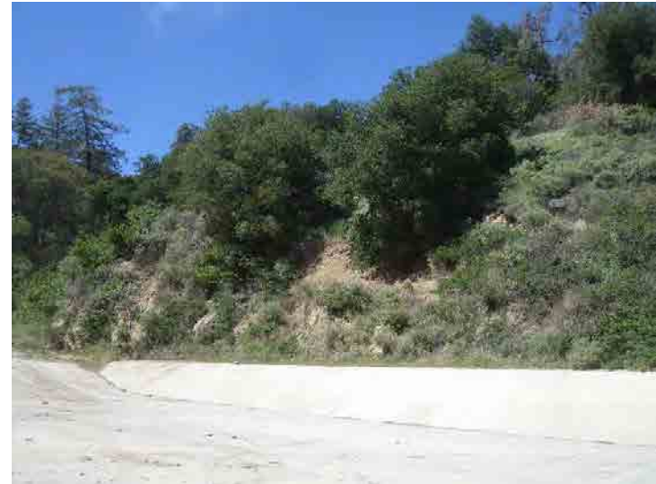
Photo 42: Basin A Native Hillside: March 23, 2016
