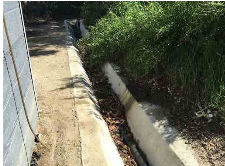
Photo 504: Leachate Treatment Facility: March 9, 2016
