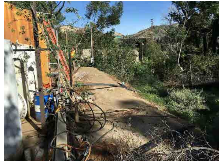
Photo 500: Leachate Treatment Facility: February 24, 2016
