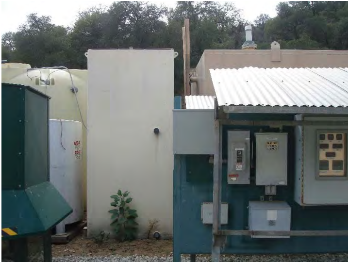
Photo 61: Condensate Equipment in Storage Yard: October 28, 2015
