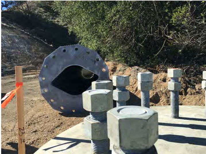
Photo 275: Edison Westside Ridge New Pole
