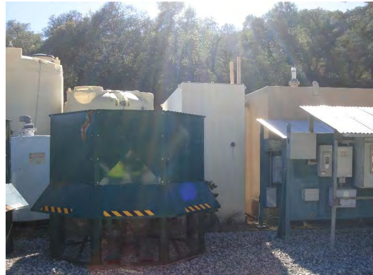
Photo 64: Condensate Equipment in Storage Yard: November 11, 2015
