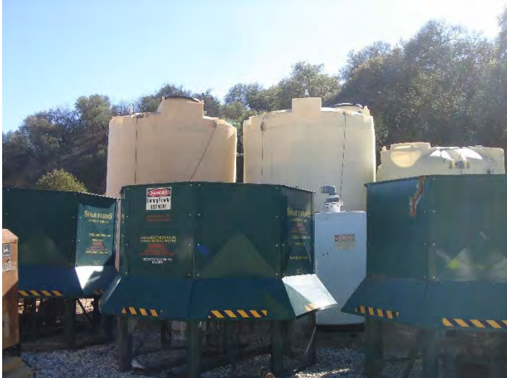
Photo 63: Condensate Equipment in Storage Yard: November 11, 2015
