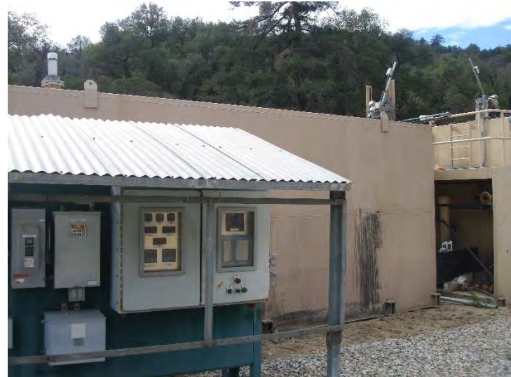
Photo 62: Condensate Equipment in Storage Yard: October 28, 2015
