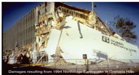
Damages resulting from 1994 Northridge Earthquake in Granada Hills
