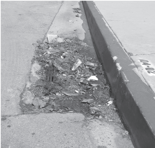
Drain clogged with debris
