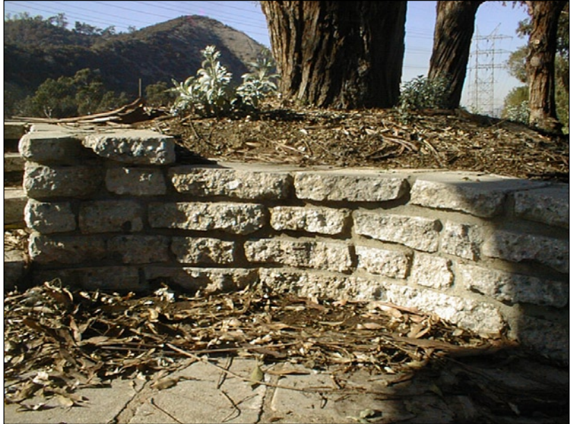
Figure 14.34 Broken concrete seatwall at Los Angeles Riverwalk at Los Feliz Boulevard, City of Los Angeles.
