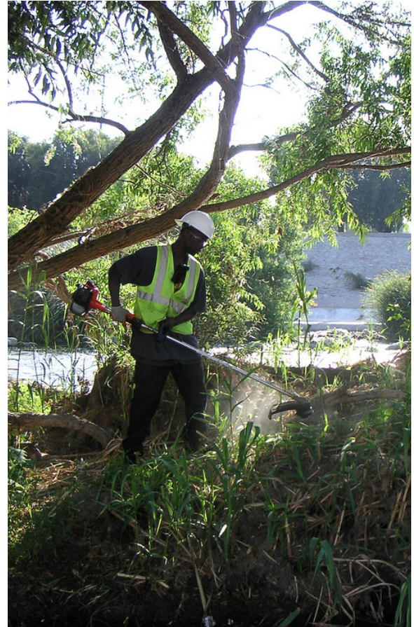
A worker removes invasive plant material from the channel near the Glendale Narrows, a maintenance practice that helps to increase the flood capacity of the LA River. Source: US Army Corps of Engineers, LA River Arundo Removal, 2004.
