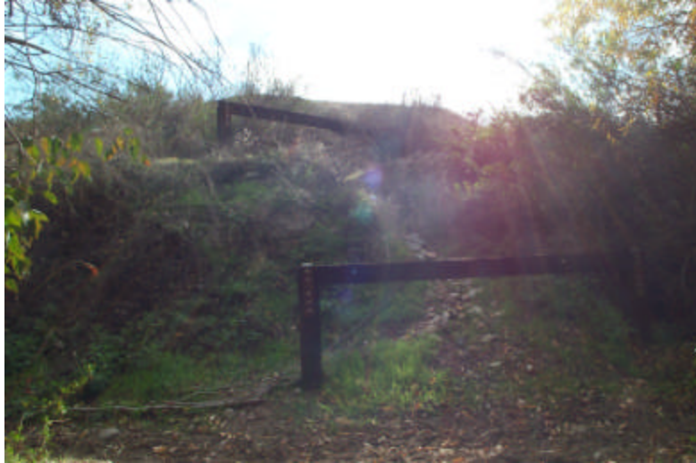
Figure 8-3a: Railroad ties used to repair the erosion gully below the Cottonwood bluff.
